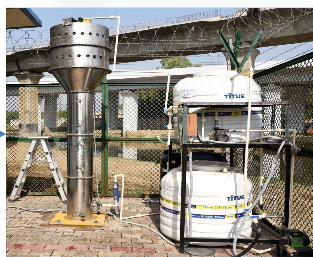
Modified Trickling Filter
